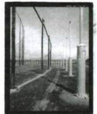
25 ft high-band reflector screens on the left, behind the high-band monopole antenna at right.
