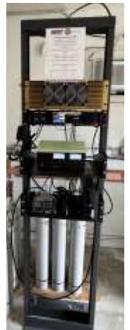
Repeater with post-amp installed.
