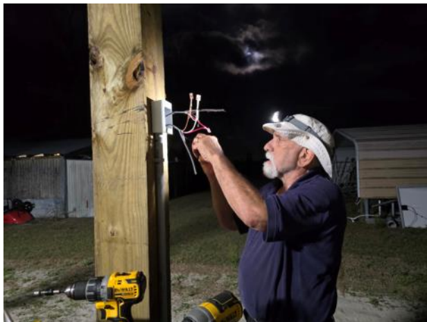
Gordon and Nancy's friend Rich (still NOCALL after 45 years of prodding) helped with the wiring while Gordon did all the digging around the 25x40 foot concrete pad!
