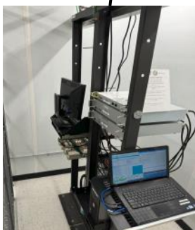
MERT's equipment in the new Marion County Communications Bldg.
