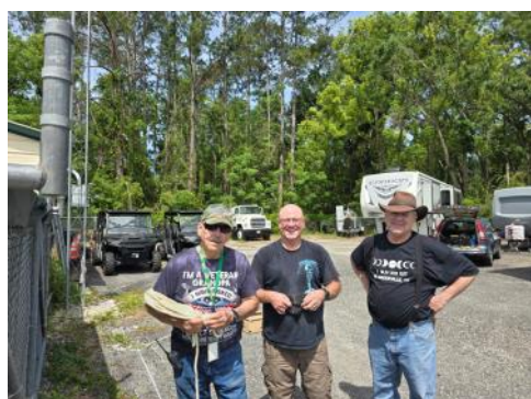
Mike KM4BTW, Randy KG7QNK and Mark KN4FRM during the installation of the new fan dipole. (Not shown is Gordon W2TTT).
