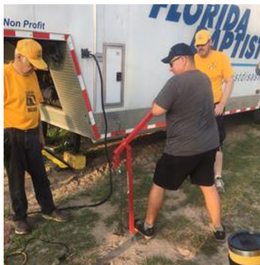
What a great idea! Small modification of typical metal fence pole puller allows ground rods to be levered right up.
